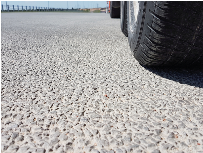
Fig. 7. The macrotexture view of exposed aggregate two-layer concrete pavement constructed in wet-freeze region for heavy trafficked transnational highway [6]
