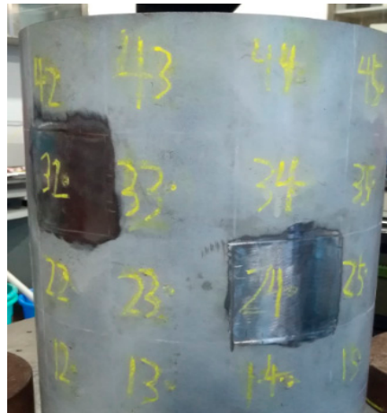
Figure 13. The damage of tank.
